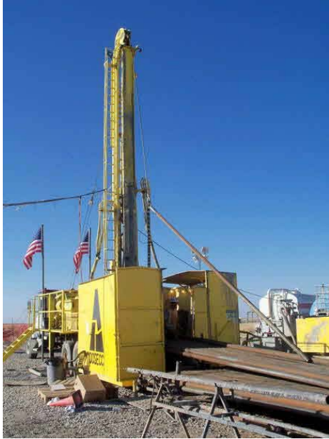
Figure 6: Pipe Tripping at the Kimberley site
